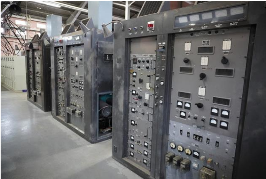
Some of the many transmitters on floor 2 at Building 2 in Bolinas.
