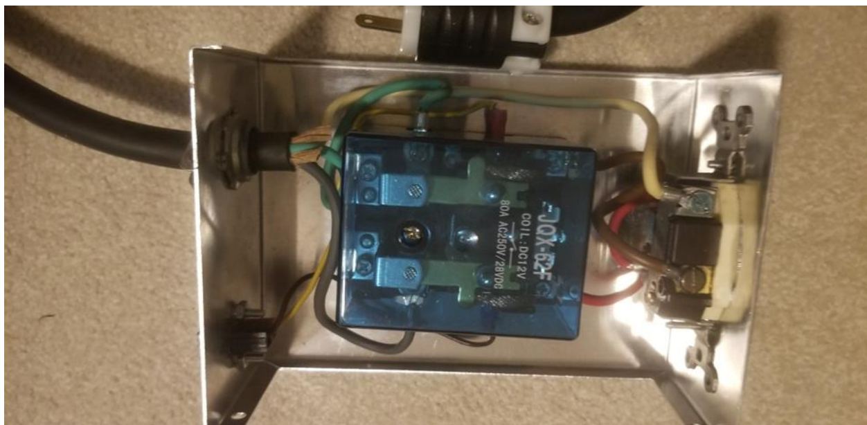
Figure 3. The completed 240 vac relay box.
